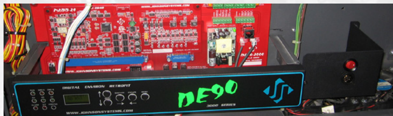
Upgraded Strand Digital Environ DE90 Rack
