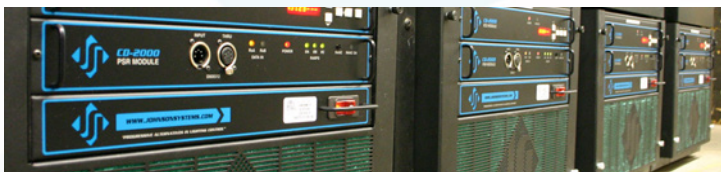
Four CD-2000+A Installed
